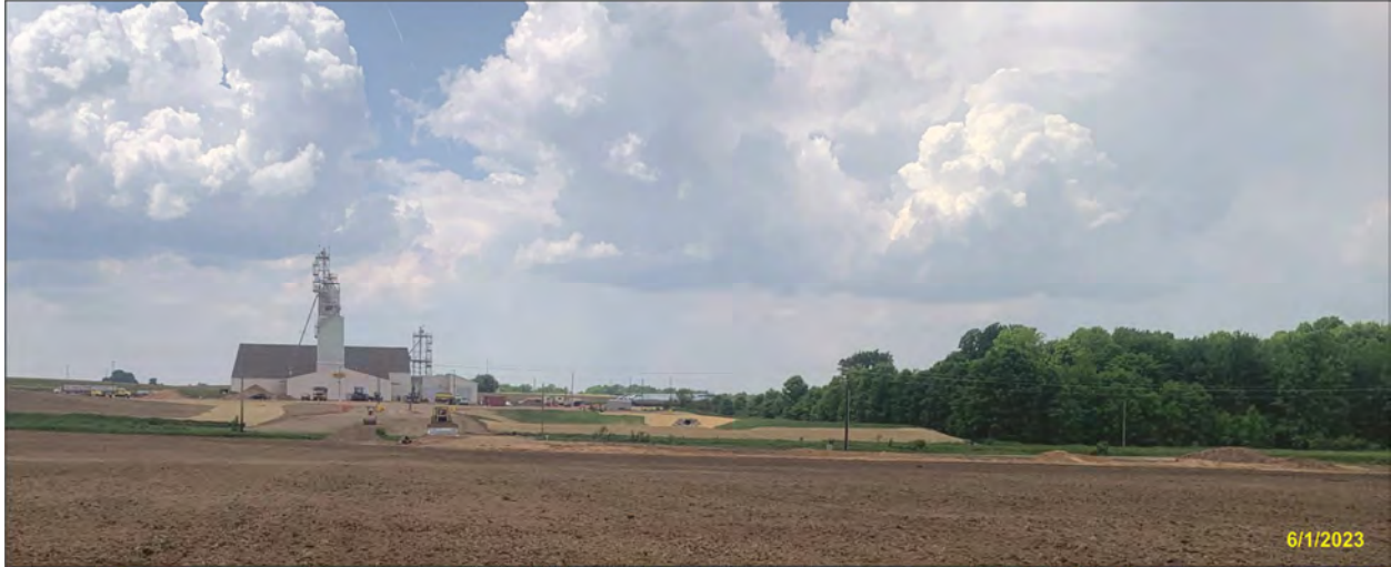
Figure 9. Part of the parcel had been graded for use as a staging area for equipment for construction on the west side of 345 th Street, shown in the background, view facing west.
