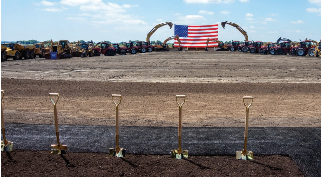
Foxconn broke ground for construction of its new facility in Mount Pleasant in June.
