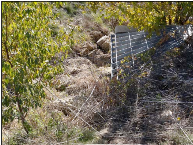
Large culvert that flows under Gateway Blvd. Note the grate at the culvert's mouth.
