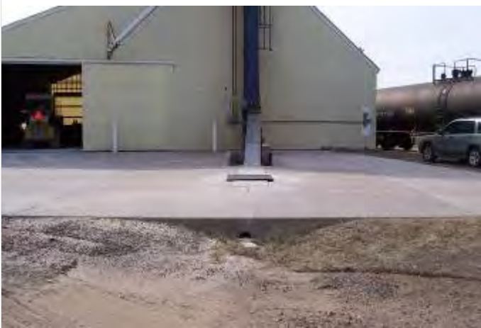
1. View of east side of load-in pad during spring event. Light colored residue is visible off edge of pad.
