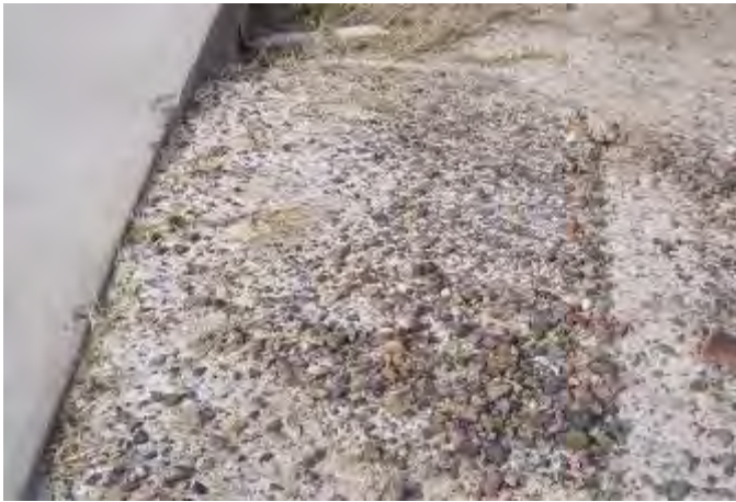
3. Additional area of residue accumulation along northwest corner of load-in pad.
